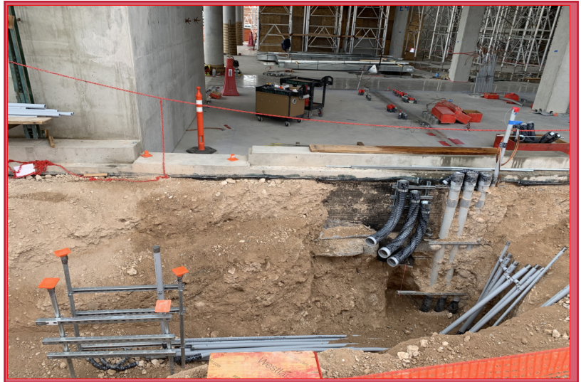
Building ATS and Generator Tie -in
