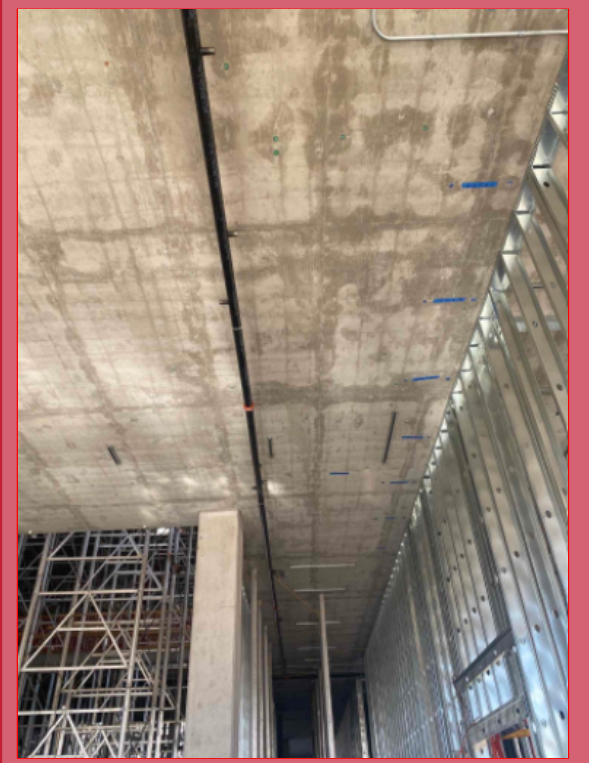
Fire Sprinkler Main Line
