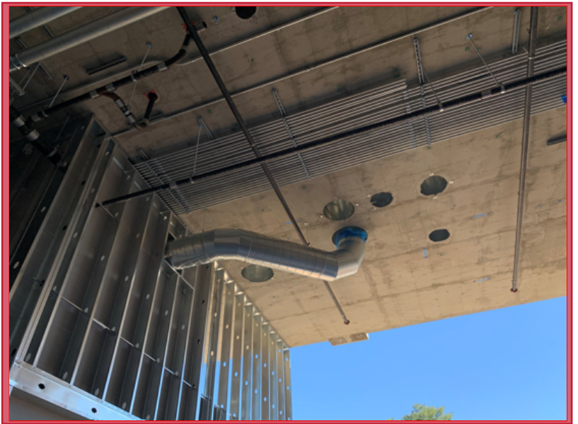
Overhead Electrical & Mechanical Duct
