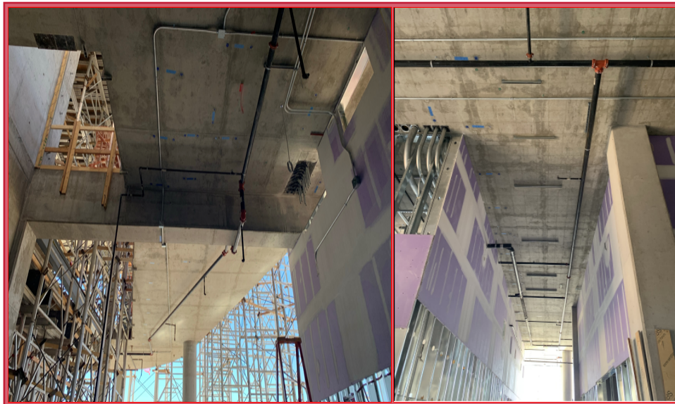
Level-1 Fire Sprinkler Main Line
