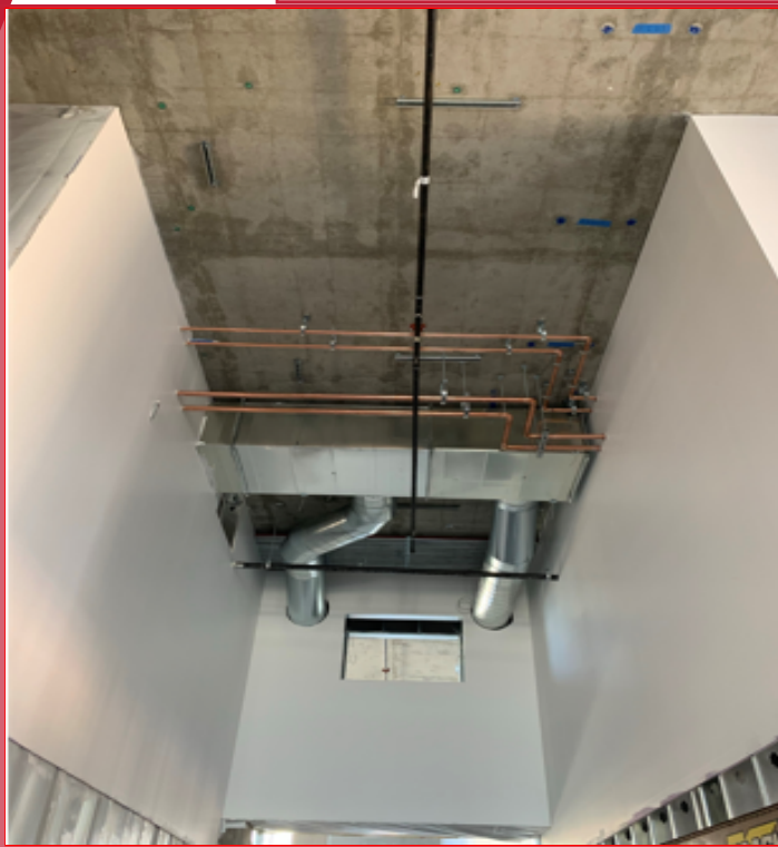
Overhead Mechanical Duct, Plumbing and Fire Sprinkler Line
