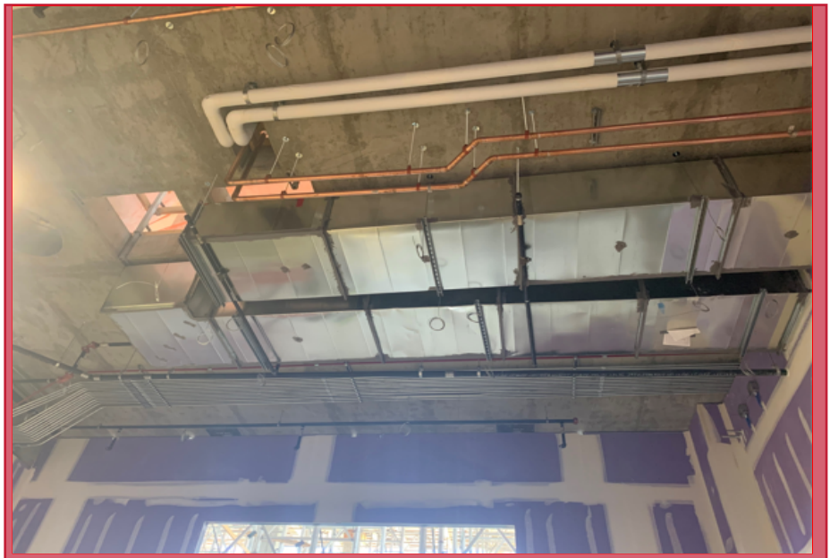
Overhead Mechanical, Electrical & Plumbing Utilities
