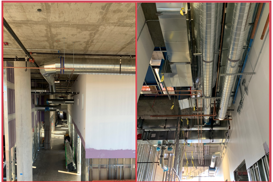
Level 2 Overhead Electrical and Sprinkler Lines
