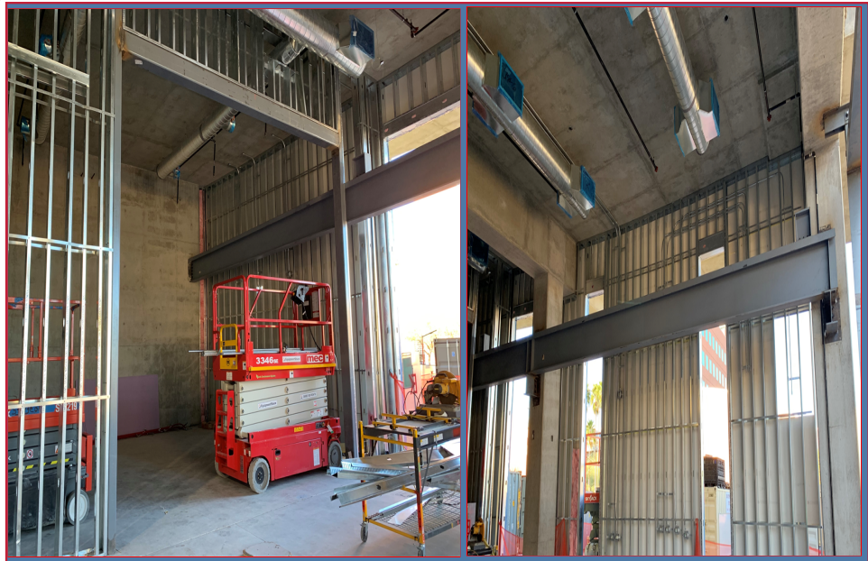
Large Scale Testing Lab Crane Steel Beams
