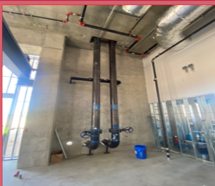
Chilled Water Risers
