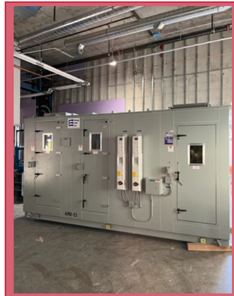
Level 2 Air Handler
