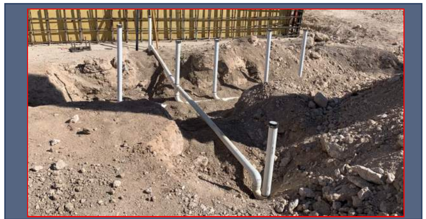
Waste Line Branches
