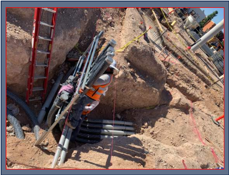
Main Building Electrical Stub-ups
