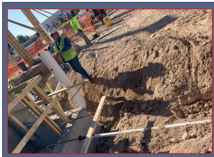
Storm Drain Main
