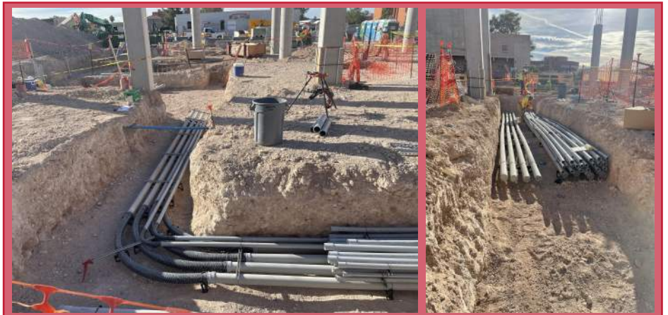
Communication and Electric Main Building Lines
