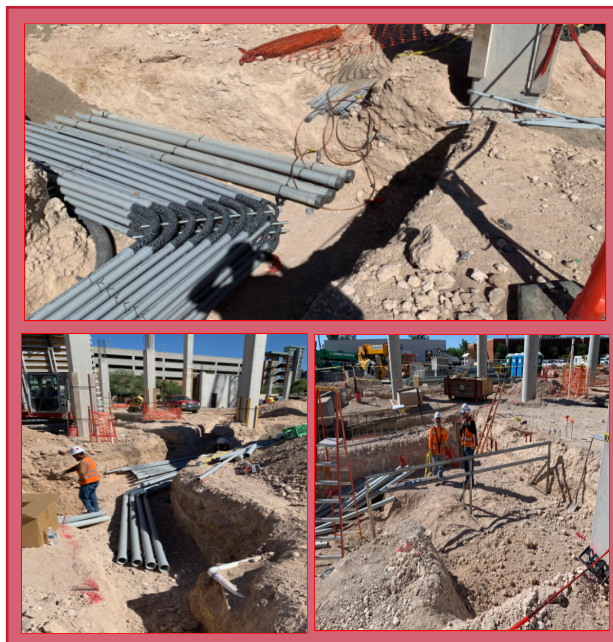
South Side UG and SES Rack Electrical
