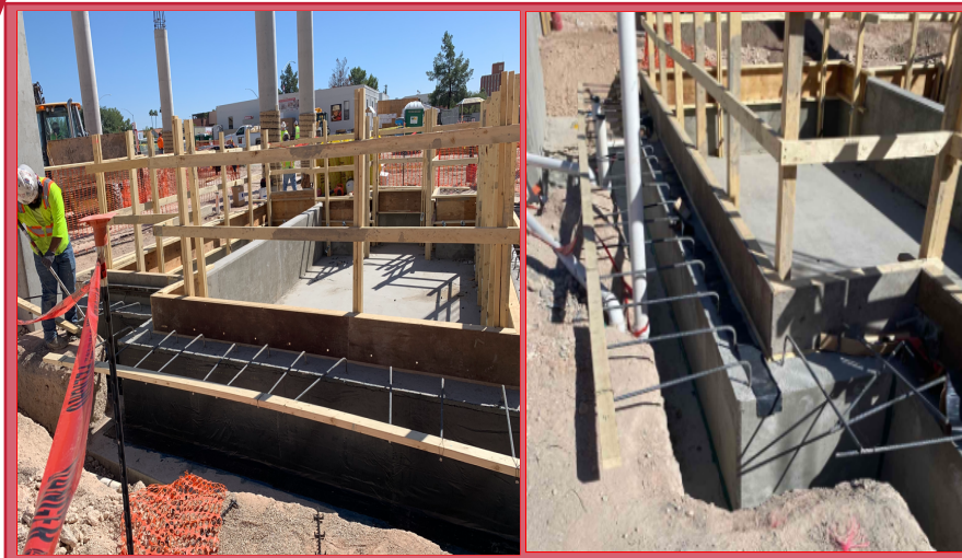
TV Chamber Membrane Waterproofing
