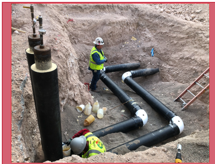
Under Ground Domestic Chilled Water Line
