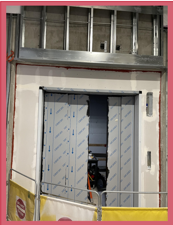
Elevator front for East elevator on level 1
