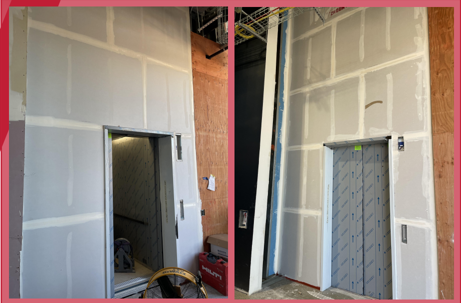
Elevator fronts for West elevator on level 1 and 2
