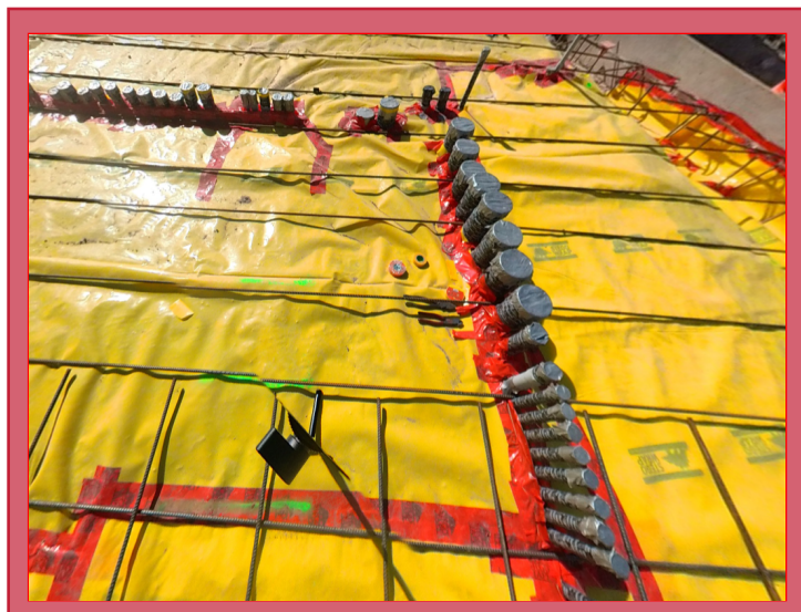
West Electrical Room Stub-ups
