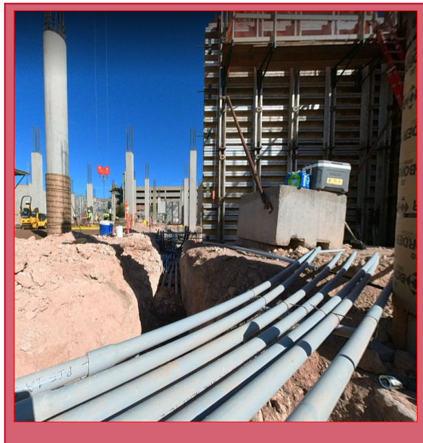
Building Main Electrical Tie-ins
