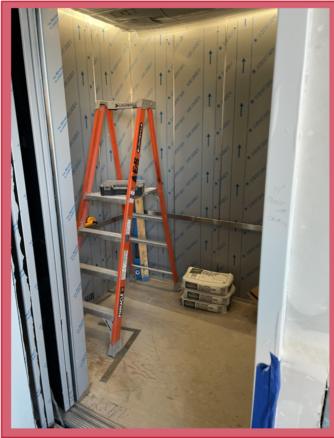
West passenger elevator serves floors 1 to 4.
