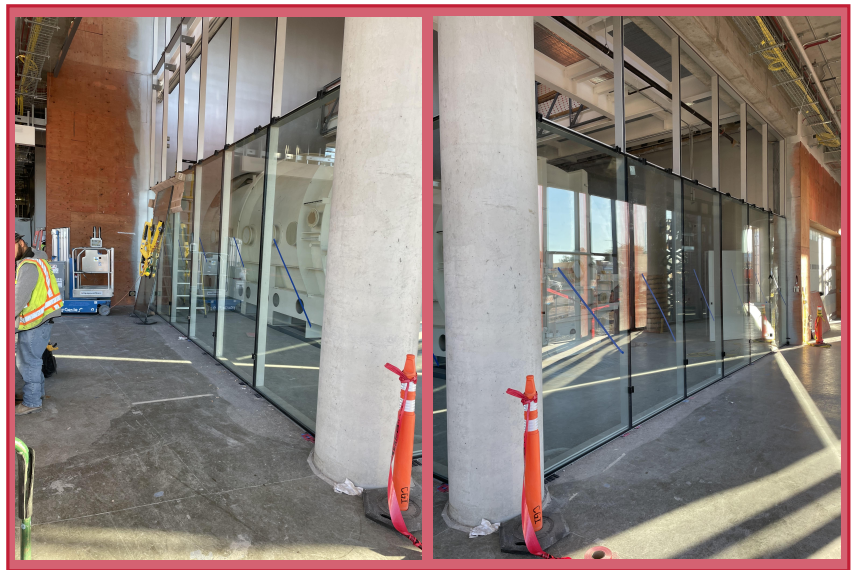
View of the curtain wall from the Southeast lobby space on Level 1
