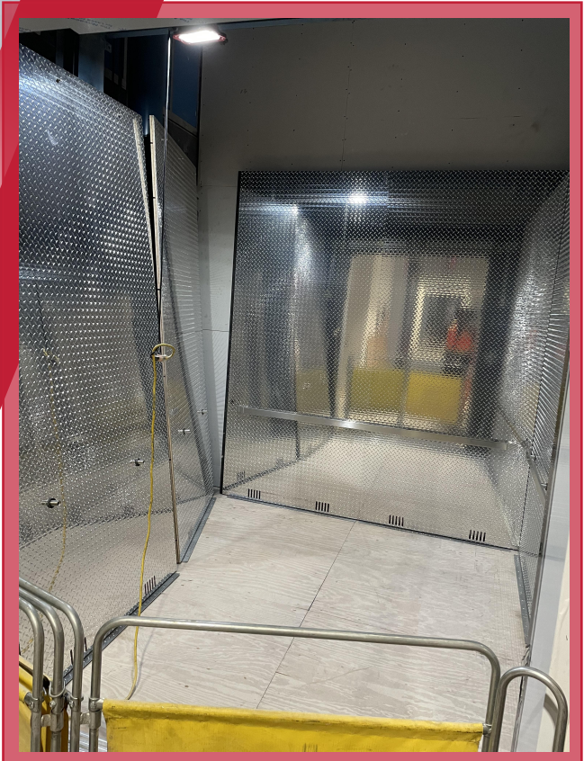
East freight elevator serves floor 1 to 3.
