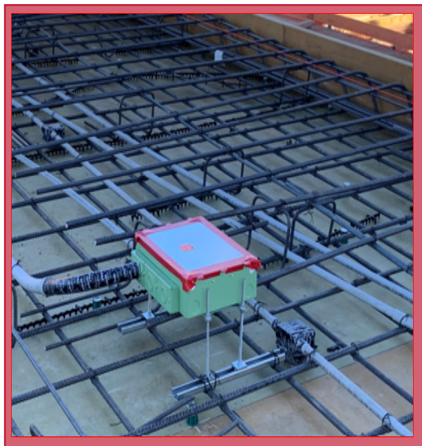
Electrical Floor Boxes On Level 2
