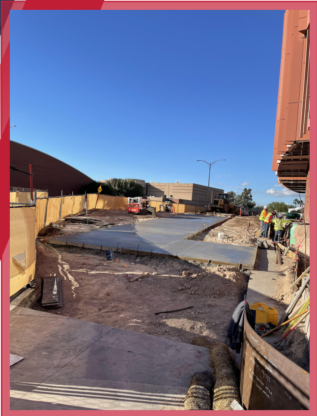
Pouring the North side of the pedestrian walkway for the Highland path
