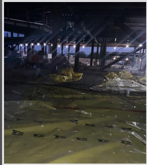
Vapor barrier and rebar displaced
