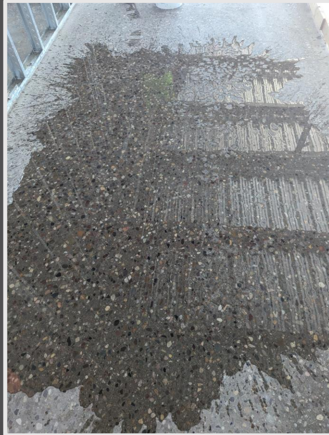
Level 2 floor with water
