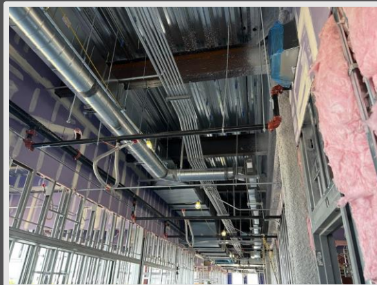
Electrical and Mechanical
