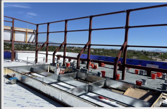
Air Handling Unit Curb
