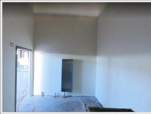
Level 1 Electrical Room
