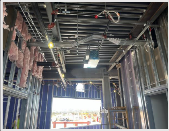
Conduits offsetting to allow for the duct work to fit as planned in the model
