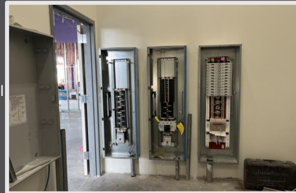
Level 1 electrical room
