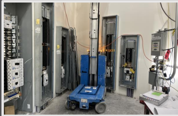
Level 3 electrical room
