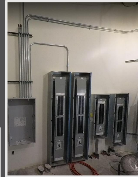
Level 2 Electrical Room
